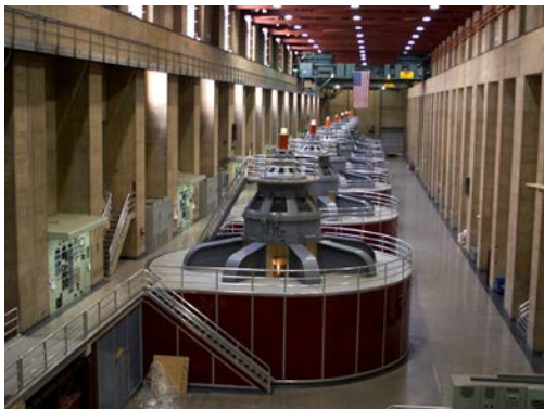
Figure 20.46 Hydroelectric generators at the Hoover dam. (credit: Jon Sullivan)
